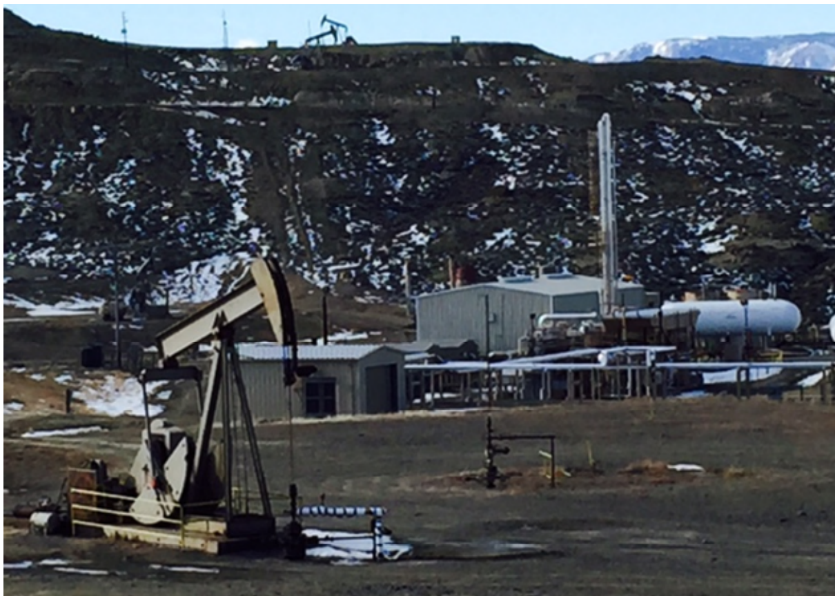
Silvertip gas processing plant
